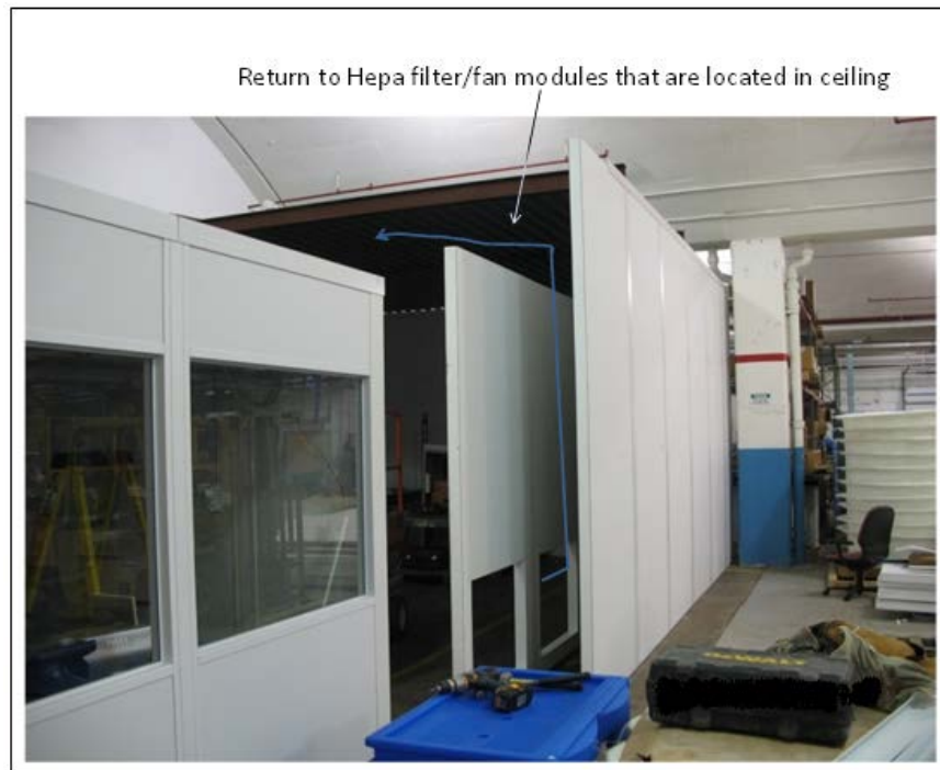
Figure 3. Photograph of return air plenum during construction. The return air plenum is formed by a double wall and ceiling; the square holes in the sidewall hold the filters.
