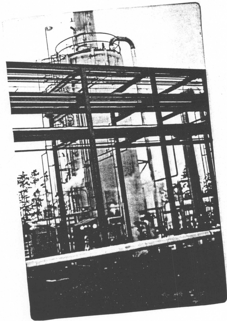
Figure 10. Slurry Preheat and Dissolving (02) Area Preheater
