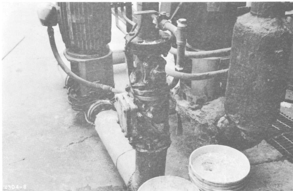
Figure 9. Absorber sampling point. Note purge collection bucket.
