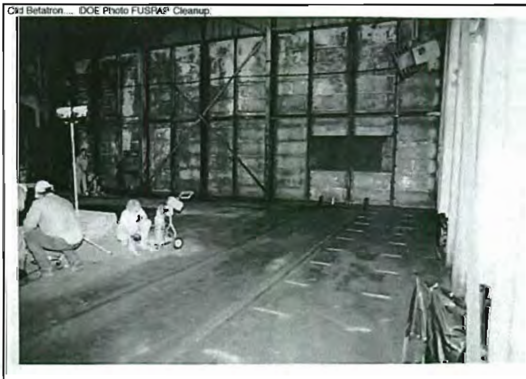
Below: By the time of the ORNL/FUSRAP cleanup 1993 most of white paint was gone
