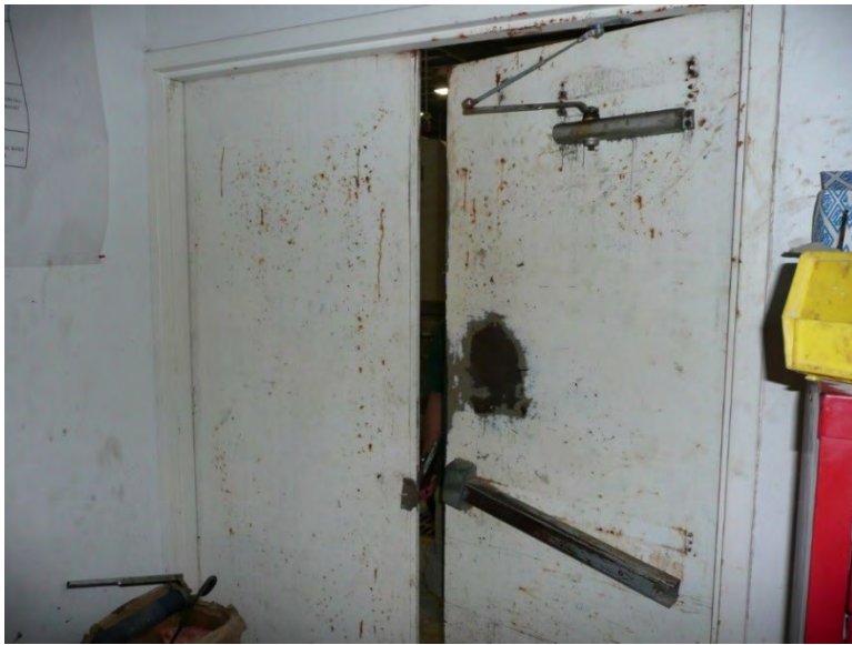
Figure 6. View of broken door from inside of the maintenance room, looking out to the production floor. Photo by NIOSH.
