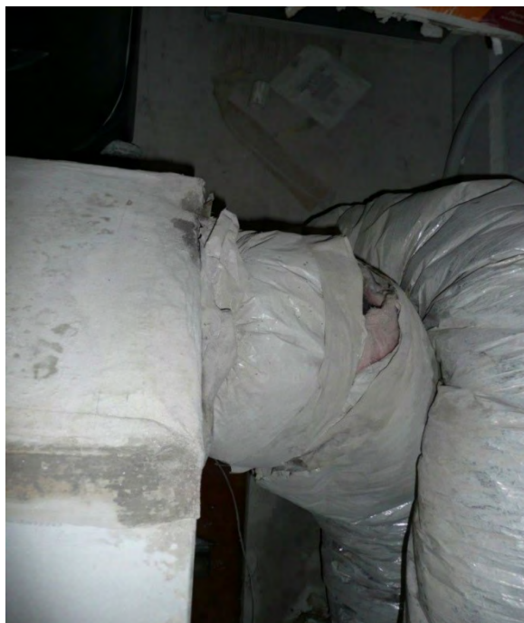
Figure 5. Torn flexible duct attached to the air-handling unit on the mezzanine. Photo by NIOSH.
