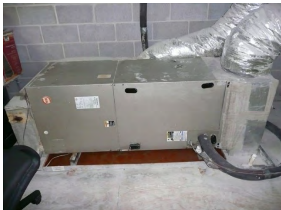
Figure 4. Discolored standing water in the drain pan of the air-handling unit on the mezzanine. Photo by NIOSH.
