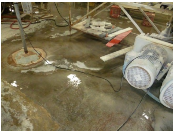
Figure 8. Electrical cords in water. Photo by NIOSH.
