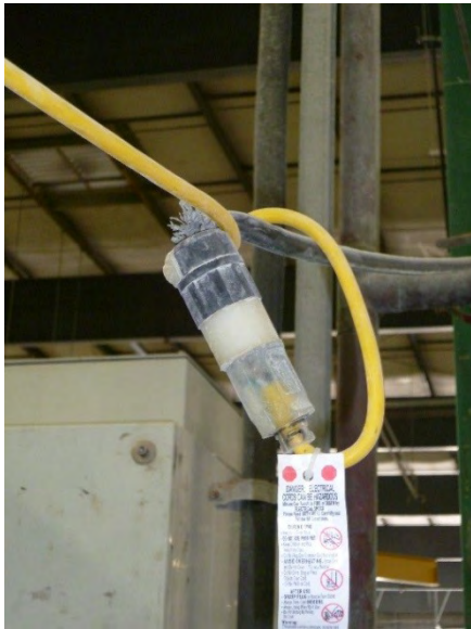
Figure 10. Extension cord with damaged insulation jacket near the plug. Photo by NIOSH.
