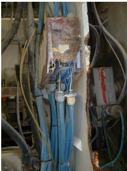
Figure 11. Severely damaged electrical junction box at Comandulli machine. Photo by NIOSH.
