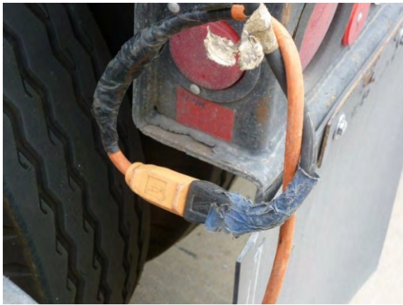
Figure 9. Electrical cords with damaged or torn insulation jackets. Photo by NIOSH.
