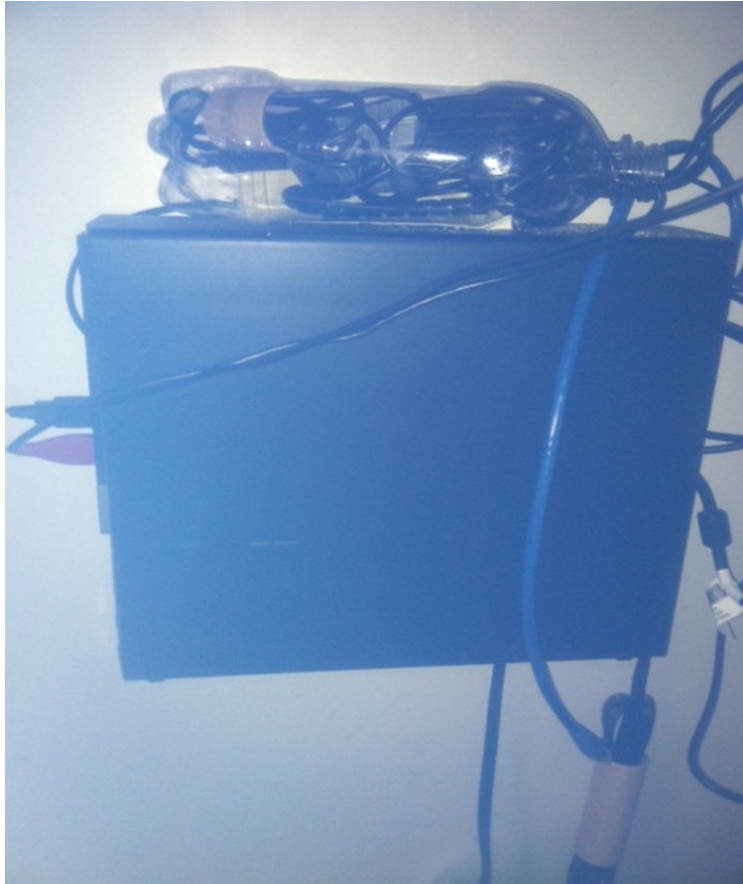
Exhibit 2-4. Small charging station under coordinator's desk
